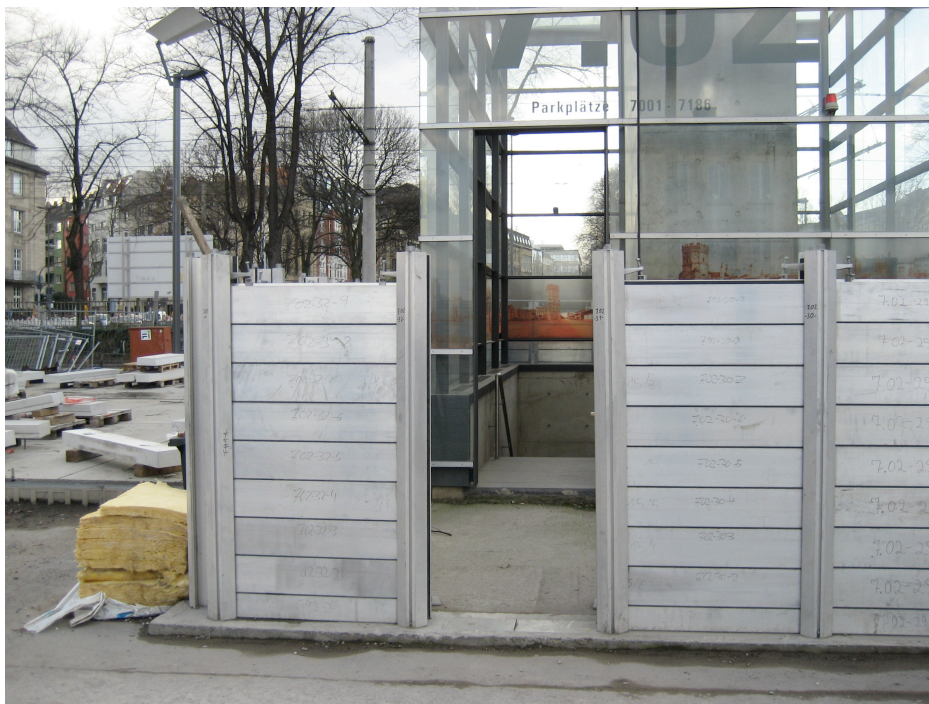
Figure 34 : Mobile flood protection sheets at entrance parking lot
